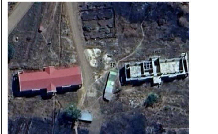
Aerial view of Buildings housing Lecture Rooms [One almost complete-roofed and another yet to be roofed], with dug out foundation plans of office building in foreground.
